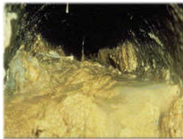
Grease buildup on the interior of sewer line.
