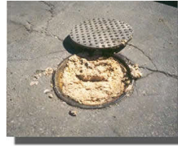
Excessive grease from overflowing manhole
